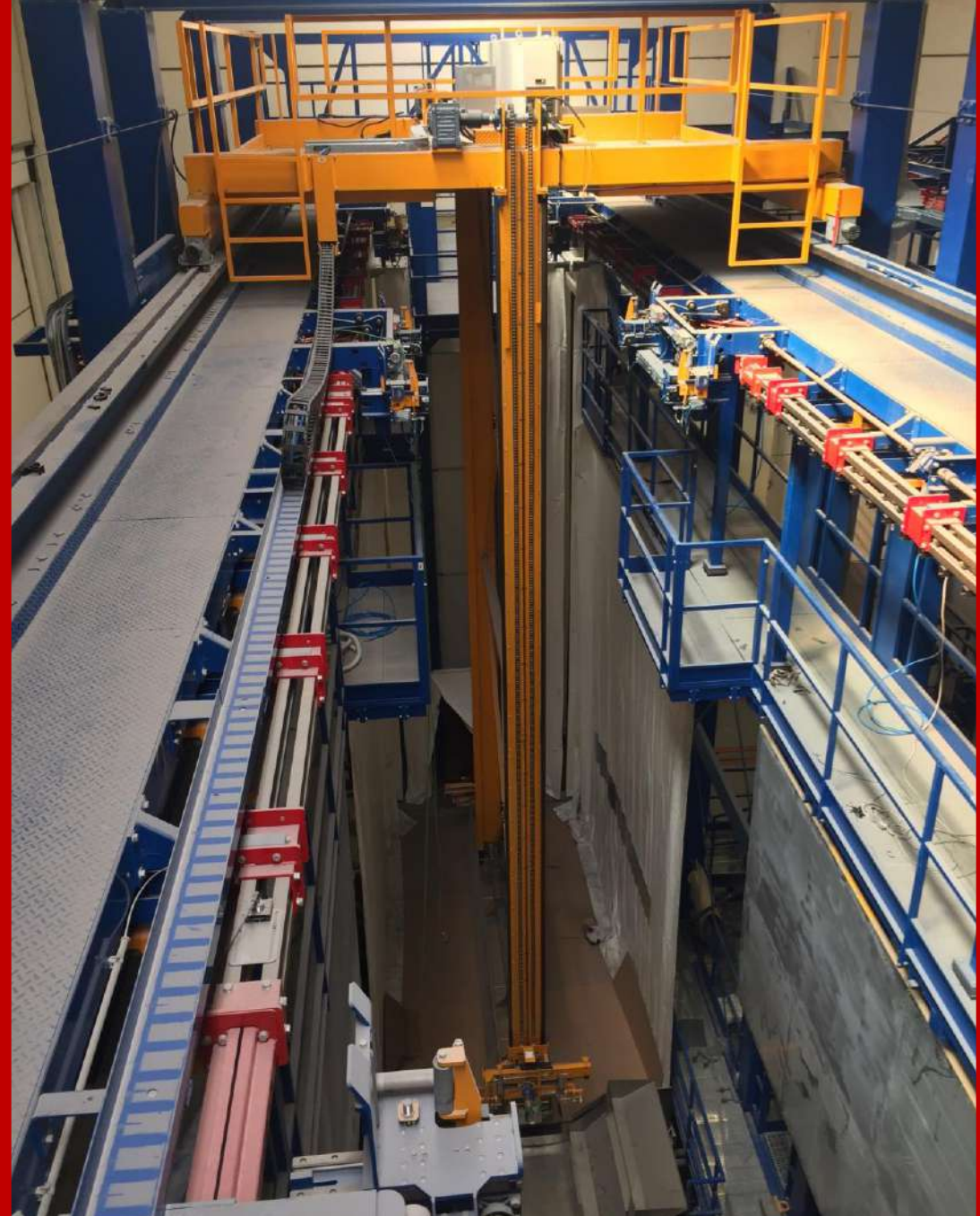
Vertical Powder Coating plant top level access aisles.
