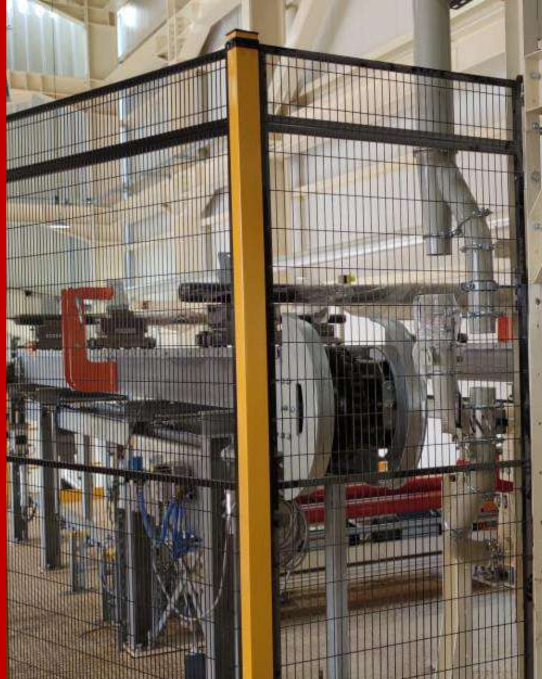
Part of the new production line.
