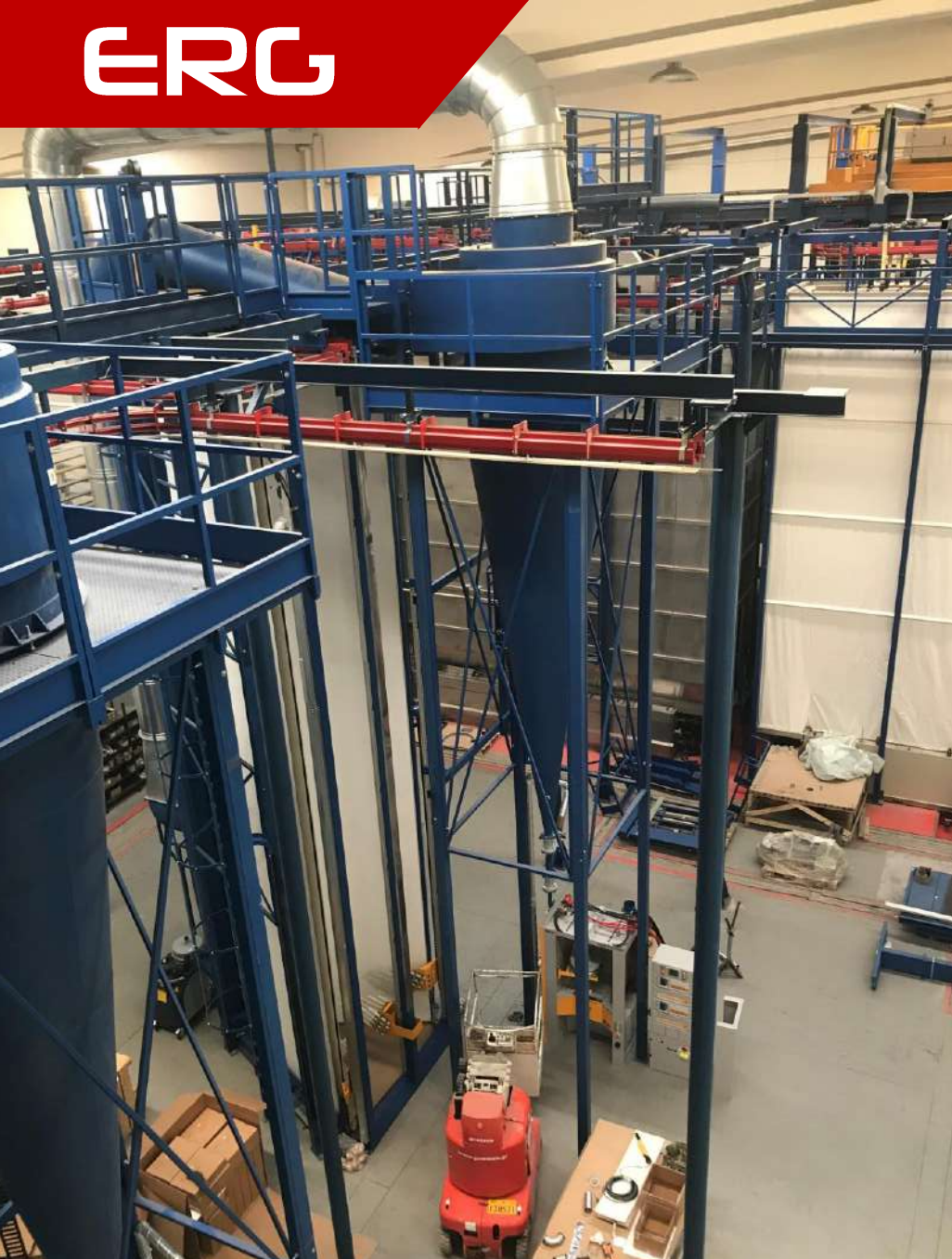
Vertical Powder Coating general plant view.
