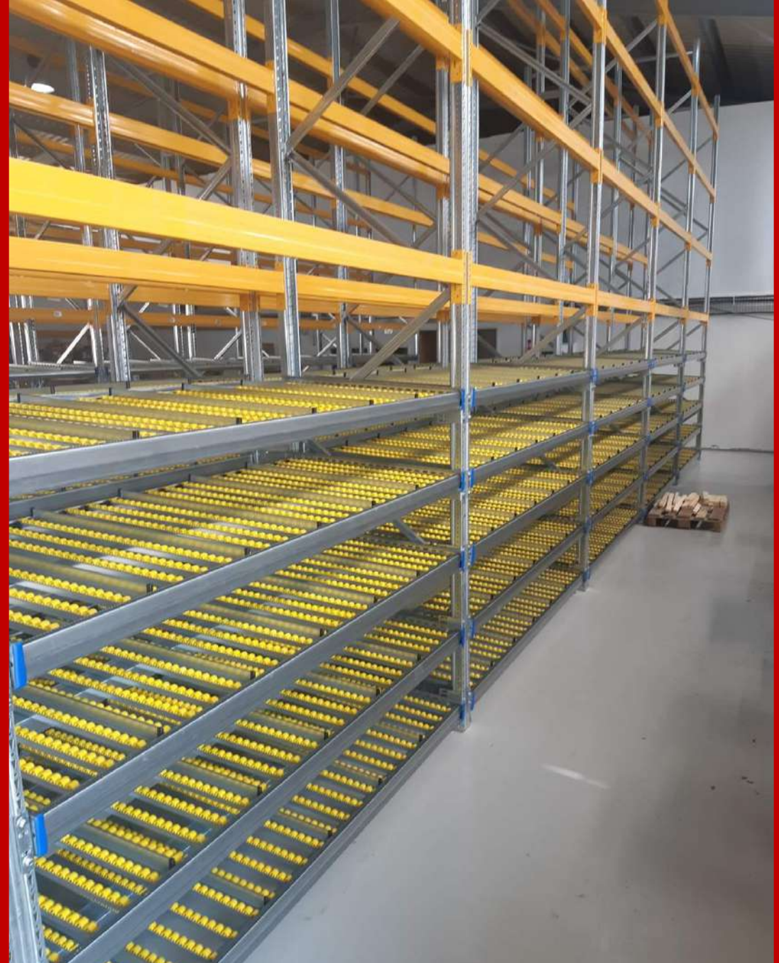
Final view of carton live storage.
