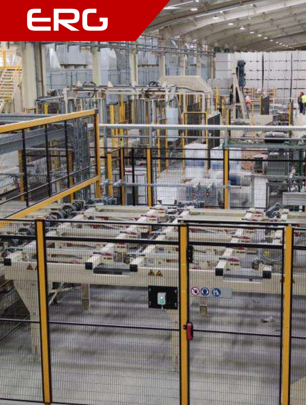
Part of the new production line.
