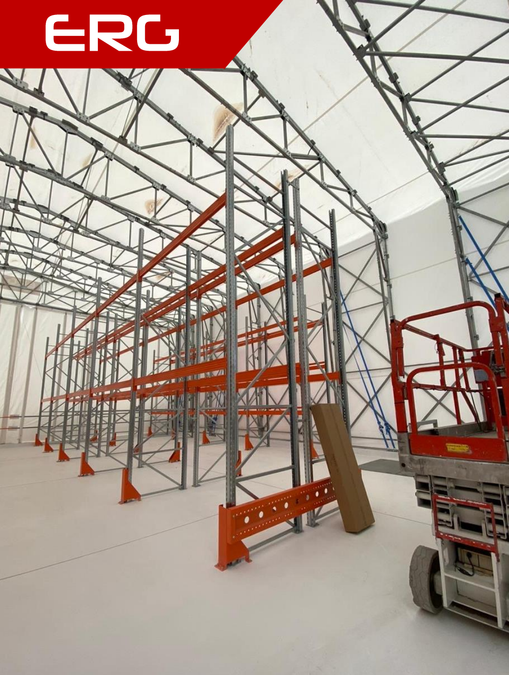
Interior view of the double mobile building with storage systems in.
