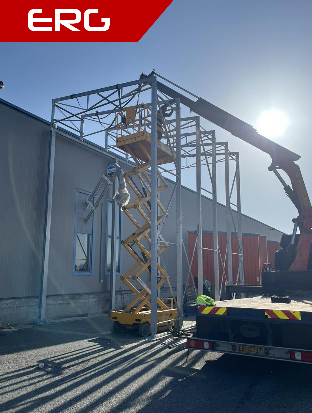
Steel structure frame with movable part of the one side.
