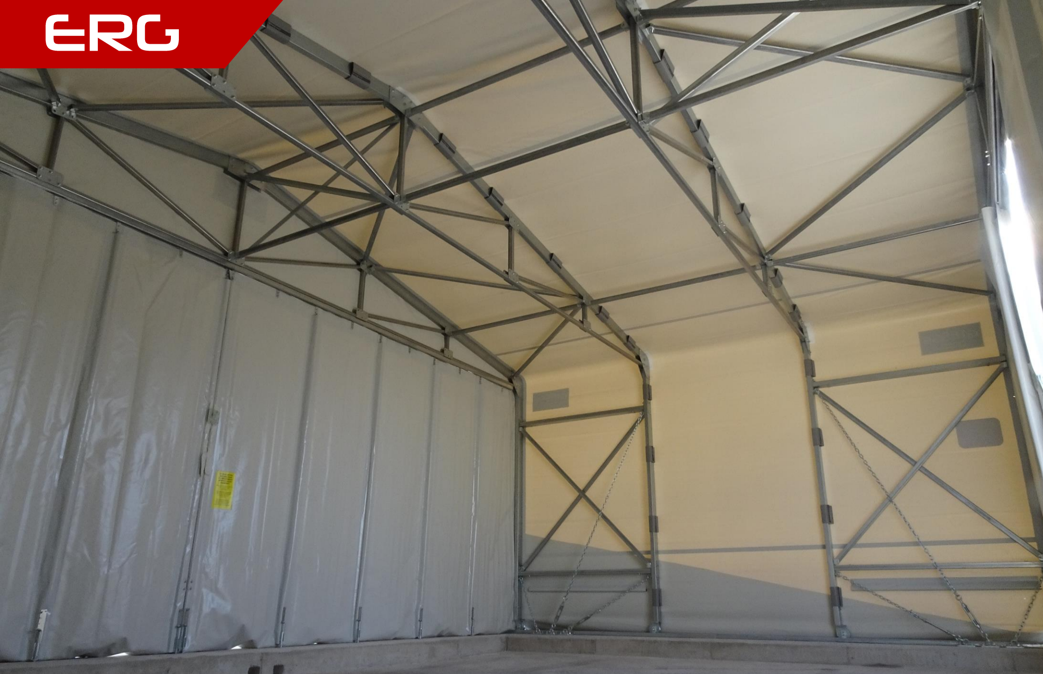
Building interior with view of the mobile drive system.
